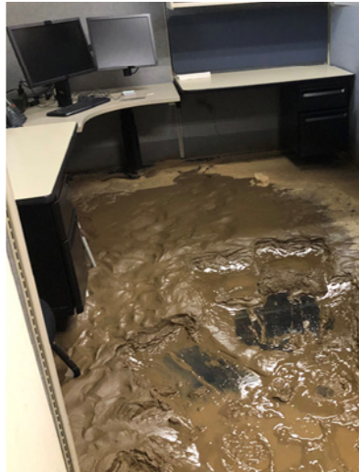
Vanguard Building Flooding
