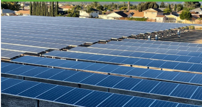
Fillmore Solar Array Farm
