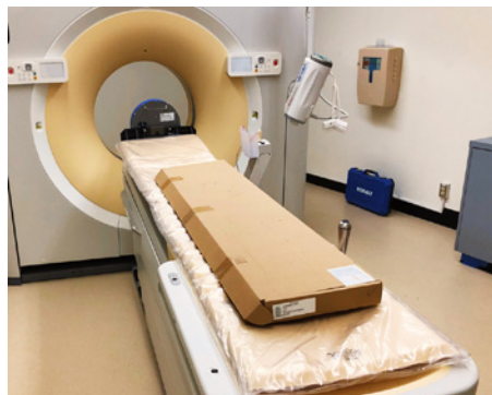
New GE CT Scanner
