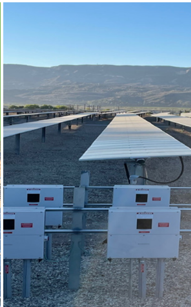
3-MW Solar Photovoltaic System
