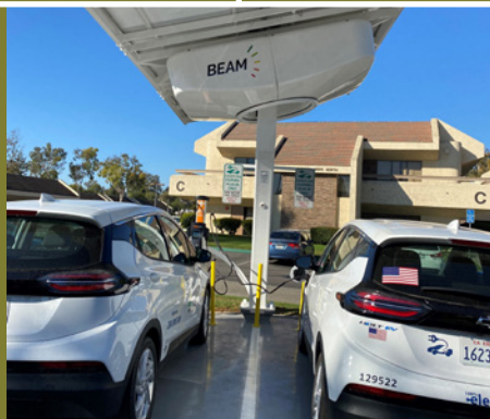
Chevy Volt EVs at Dual-Port Charging Station
